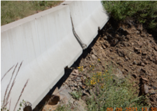
Erosion by Dave Mowry of Undercut Jersey Barriers
