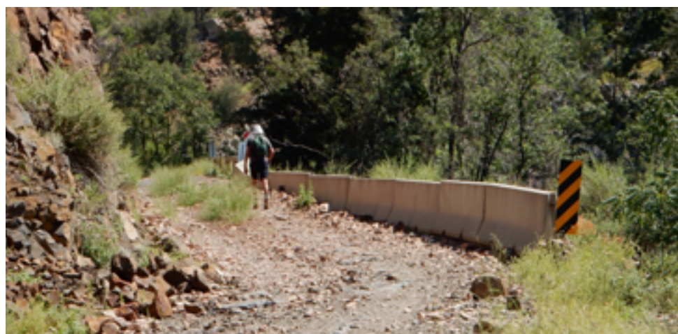
Road Closure by Dave Mowry of Undercut Jersey Barriers
