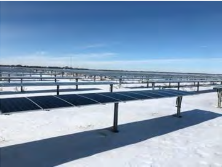
Single axis tracker system in winter.
