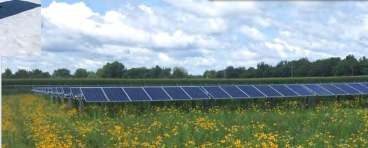
Example of single axis tracker system in summer.
