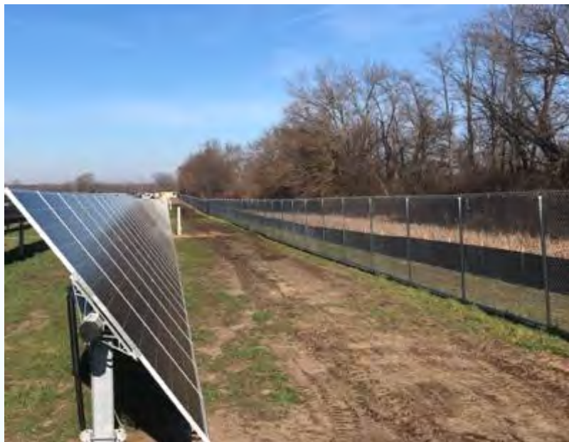
Example of chain link fence and interior road around solar project.
