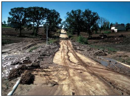
Construction site after a storm. Drift fences were not constructed to hold the soil in place. Photo Credit: Lynn Betts, USDA NRCS
