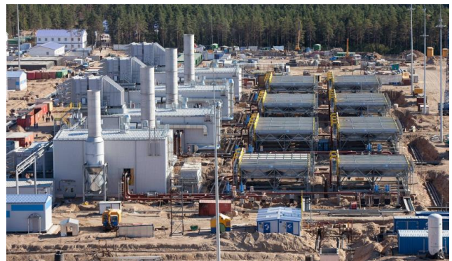
Natural Gas Pipeline Compressor Station
