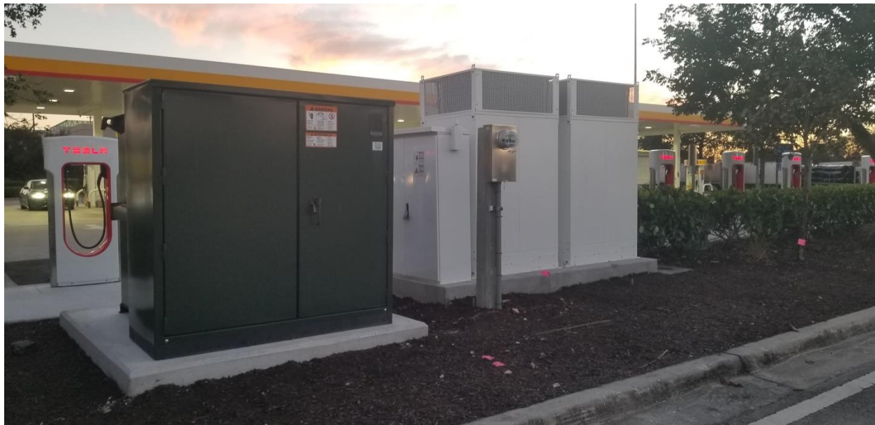
Figure 21 Electrical equipment for BEV charging station at Florida Turnpike Lake Worth service plaza from north side looking south. This area could easily be used to double the charging stations when needed. Gulf service station in the background with gasoline pumps approximately 60 feet away.
