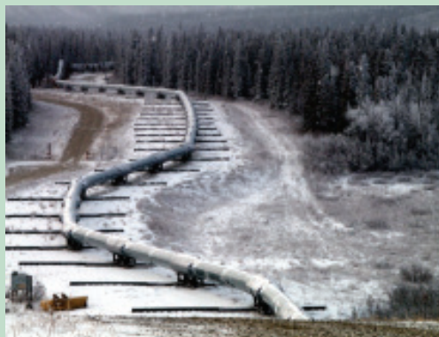
Gas pipeline repair specifications should mandate zero leakage, as should any new pipeline construction or extension.
