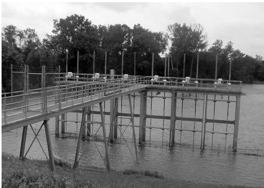
Figure 6. The St Johns Bayou gate in the set-back levee. When the Mississippi River level is above the bayou, the gates are closed to prevent backwater flooding in the St Johns Basin.
