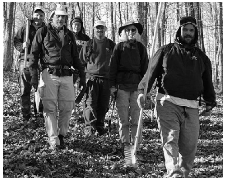
Sierra Club and Ozark Trail Association volunteers conduct maintenance and construction along the Bushy Creek section of the Trail.
