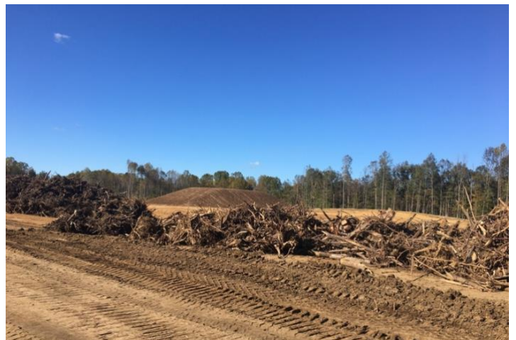
Land being cleared near Commerce Drive and Prince George's Boulevard in Bowie for sports fields.
