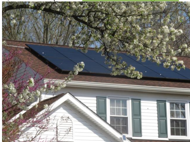
Many Prince George's County neighbors have rooftop solar arrays.
