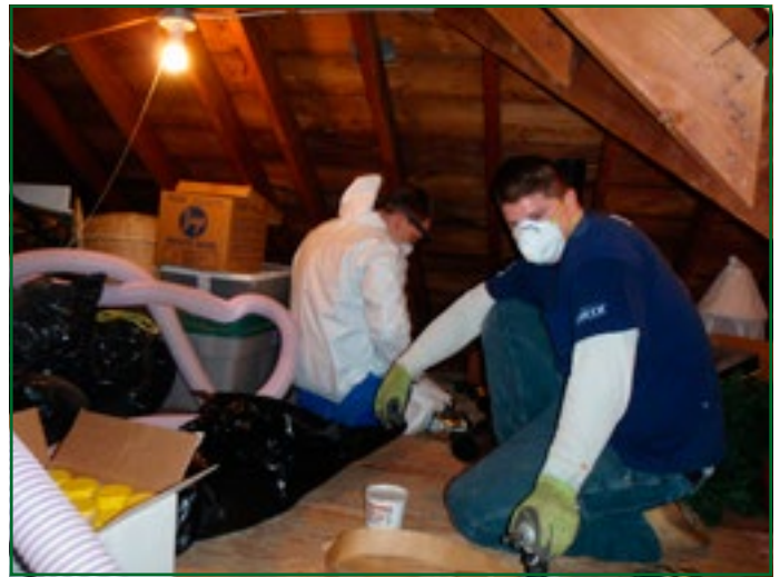
Photo by Mike McHugh. Nicor Home Services workers insulate the McHugh home.
