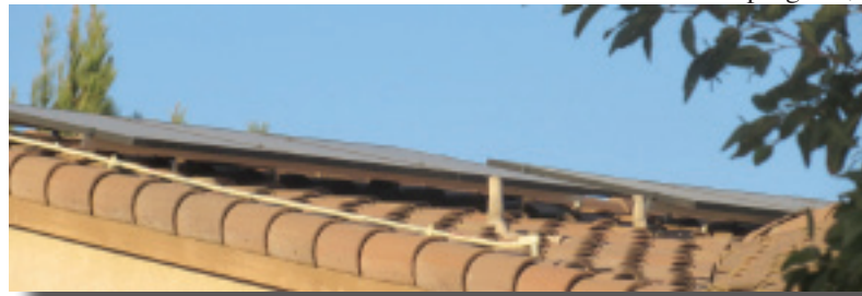
Close up of Mike's rooftop panels.
