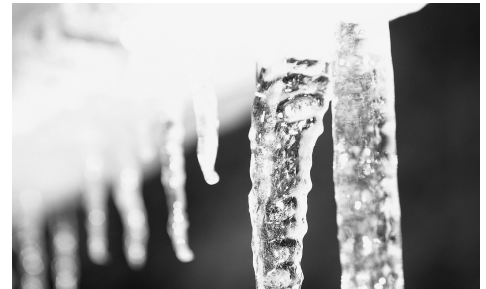
Heat loss thru a roof can cost you a lot of money and trouble.
