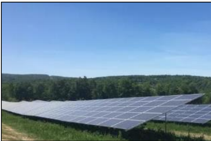
7.5 MW solar farm, Millard Hill Rd., Town of Newfield, NY. Photo: Binghamton Press & Sun-Bulletin https://www.pressconnects.com/story/news/local/2018/08/17/solar-power-new-york-state-renewable-energy/848908002/
