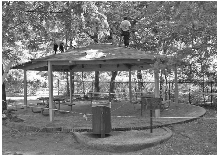
The picnic gazebo at Rozelle-Annesdale Park gets a new roof. Photo by Stoy Bailey.
