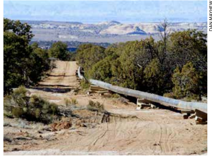
75% of the length of this pipeline will be above ground and vulnerable.
