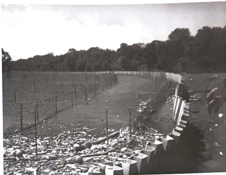
Temporary sheet piling allows planting for Anacostia wetland restoration. (photo courtesy of D.C. Watershed Protection Division)
