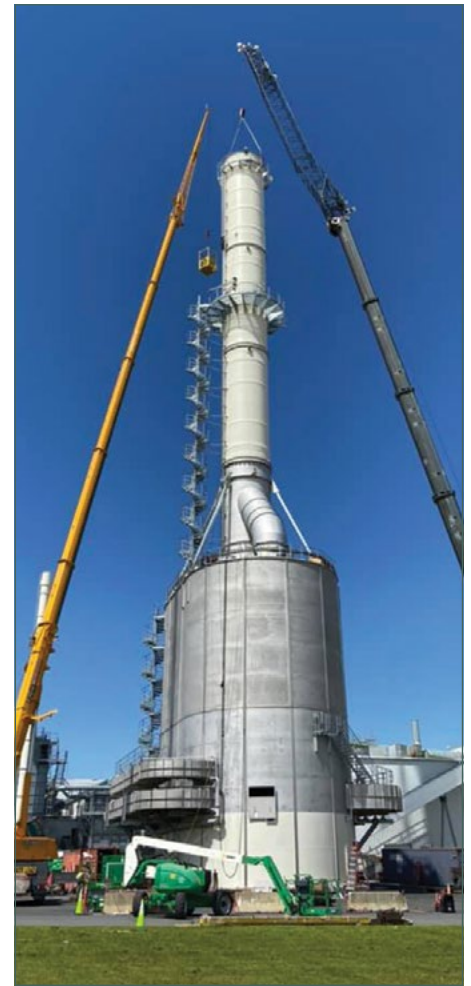
Rockwool's largest amount of particulate matter is coming off the melting furnace and those emissions do not go through the wet electrostatic precipitator control, pictured here.
