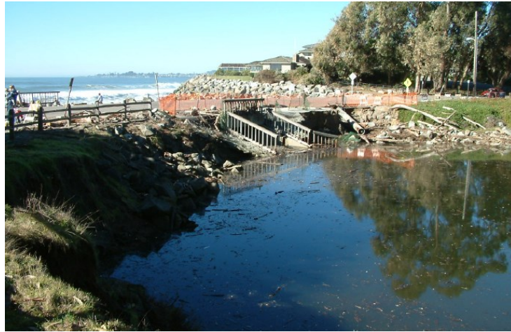
Moran Lagoon road crossing on East Cliff Drive, with a single culvert which constricts breach location, and significant weight placed upon the rest of the original lagoon frontage.
