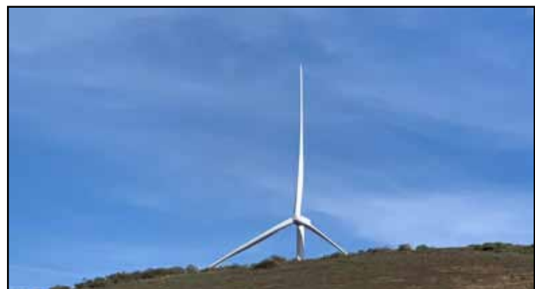
Wind turbines are being erected along Lompoc-area hills and coming online fast, expected to power on in 2023. The Strauss Wind project will provide enough energy for 44,000 homes. (Photo by Rick Skillin)
