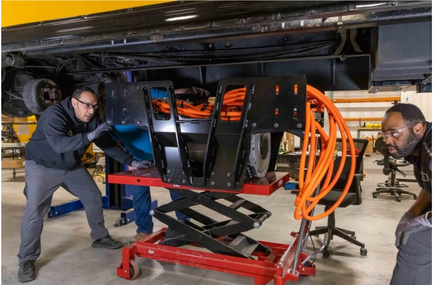
As part of the repower process, technicians install an electric motor and high-voltage cables between the school bus chassis frame rails. Photo by SEA Electric.
