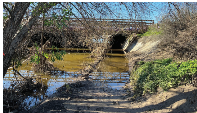
Palo Alto Baylands underpass during King Tide.
