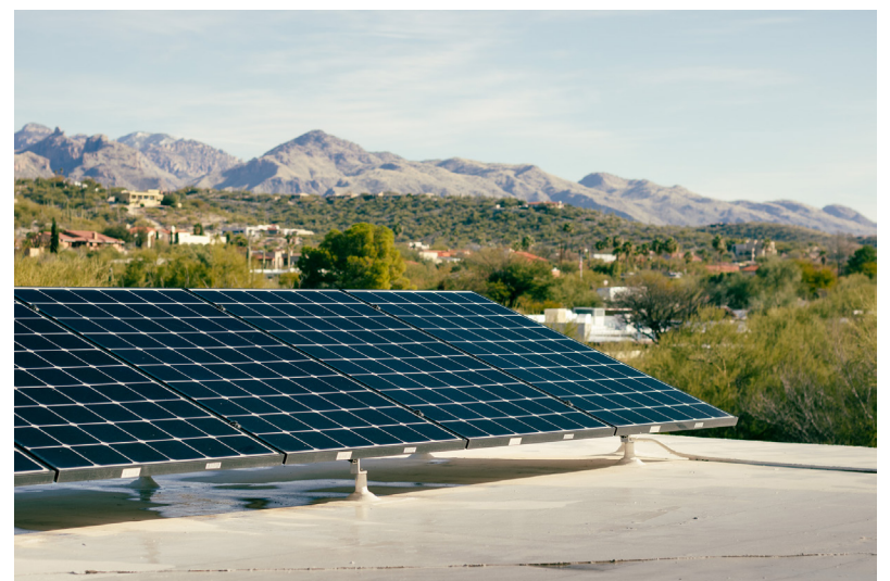
Residential Solar Installation. Photo by Adrian Keller.
