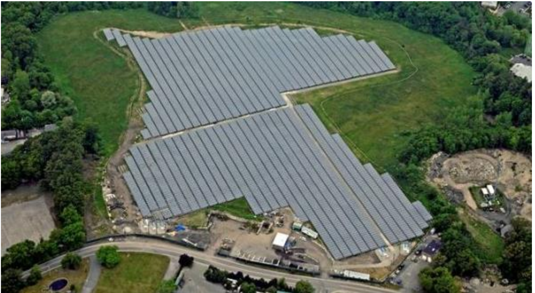
Canton, MA: 15 acres of panels on 40-acre landfill; 5,750 kW
