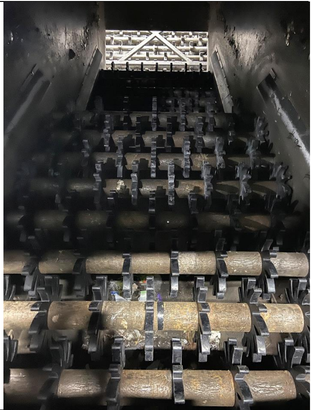
The screens after cleaning
