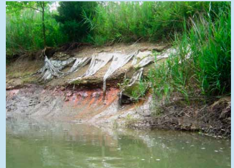
THIS STEEL CAGE OF ROCKS BACKED BY A GEO-TEXTILE LAYER WAS DESIGNED TO PROTECT THE RIVER FROM THE ASH PIT. EVEN THE SIMPLEST OF STRUCTURAL CONTROLS HAS FAILED AT THE VERMILION RIVER SITE.
