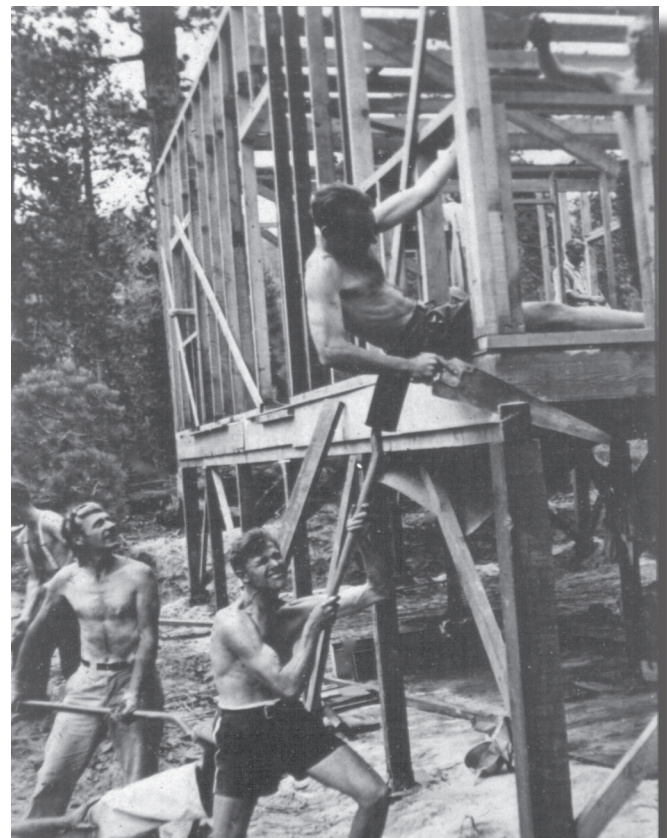
Howard Gates supporting Howard Koster during building of Keller Ski Hut, 1938. [Muir Dawson Collection, Angeles Chapt. Archives]
